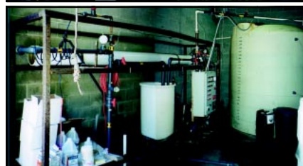
Ultrafiltration Treatment System.
