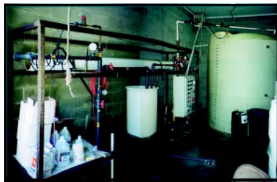
Ultrafiltration Treatment System.
