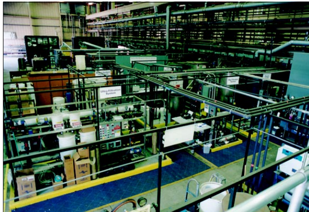
Package Plant Area
