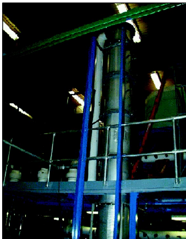
Figure 3 - Pilot-Scale Air Stripper Column.
