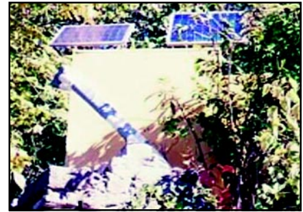
Data Collection System with Solar Panels.
